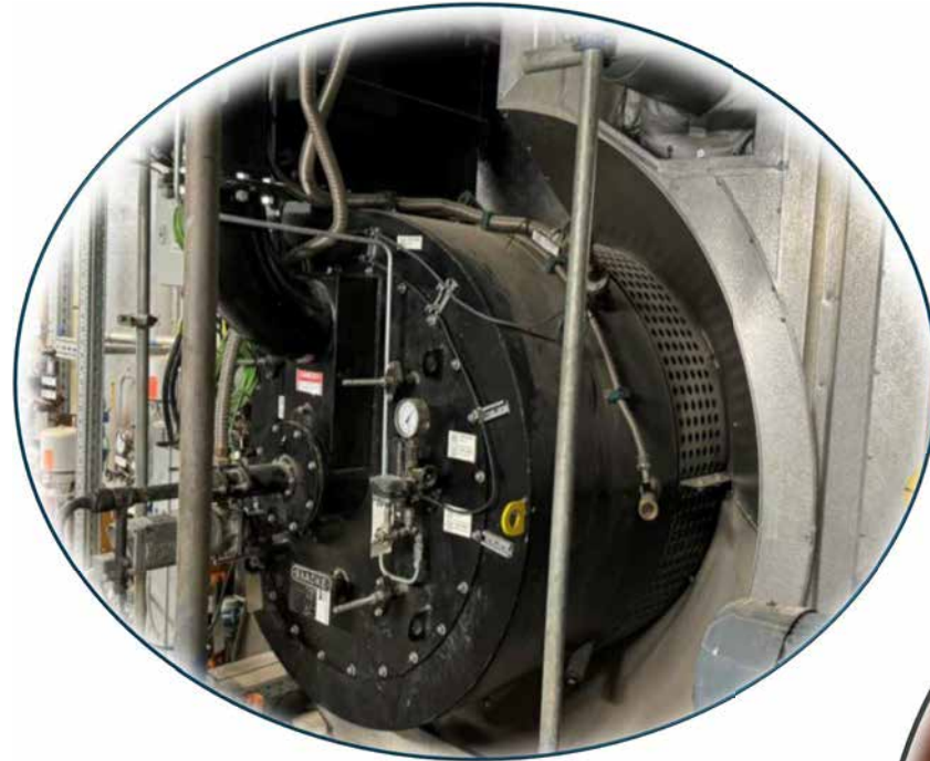
SAACKE SSB Burner on site
